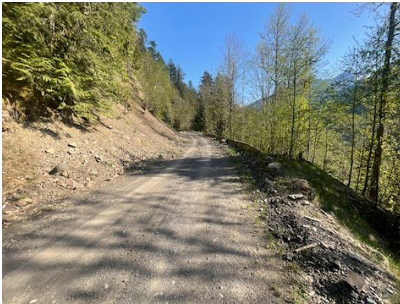
Town approach, unstable upslope.
