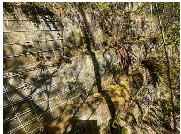
Failing layer in bottom grs system.
